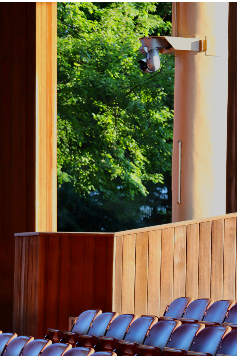
HR140 cameras are mounted on custom designed brackets and attached to the stage walls, and in front of and on the balcony.
